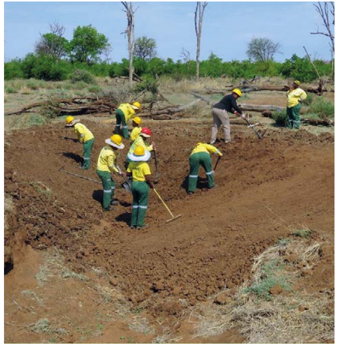
Reshaping of the gully (J Buckle).
